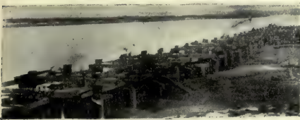
FIG. 129.—Revetment in the Missouri River to prevent undercutting. The river is flowing from left to right.
